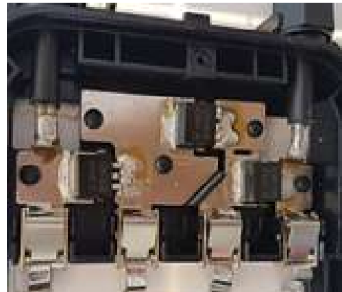
Fig. 3. SP connection diagram (above); Photos of the shunt diodes D0 in the junction box from the back of the SP (below)
